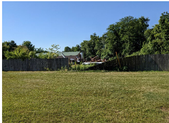
Screen fence with Road District maintenance yard has collapsed in several locations.
